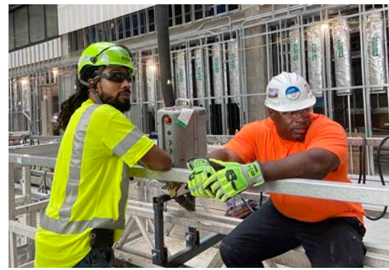
Michael Brown (left), Summit Anchor project manager, sports a high-visibility helmet with an integrated visor while consulting with Tyrone Powers (right), Spider technician, at a project in Washington, DC, in August 2022. Powers is wearing a traditional construction hard hat.
