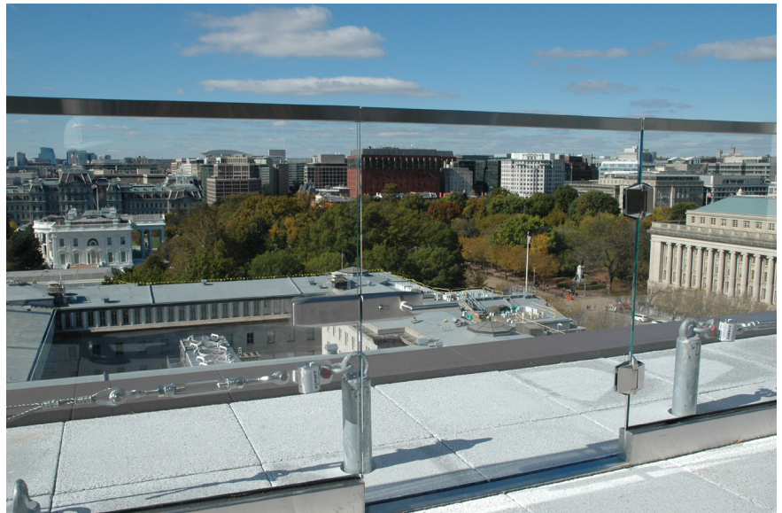
Figure 9 - HLL designed in conjunction with an access gate. Note that HLL was interrupted to reduce a trip hazard when walking through gate.
